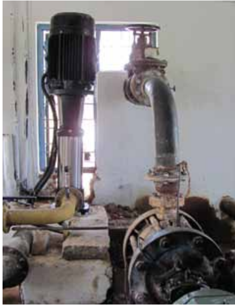
Improved pumping machinery
